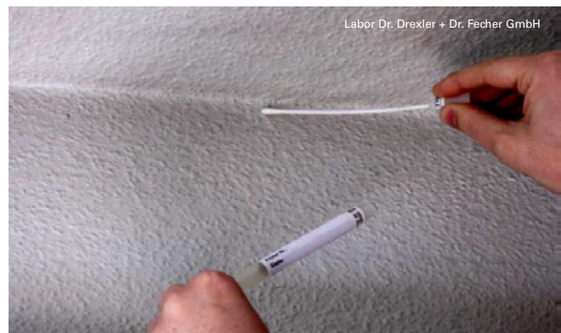
Material-Check: Schimmel Abstrichprobe.
